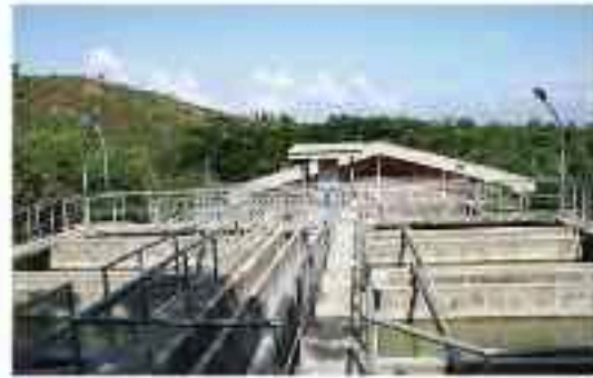
Water Treatment Plant (WTP)
